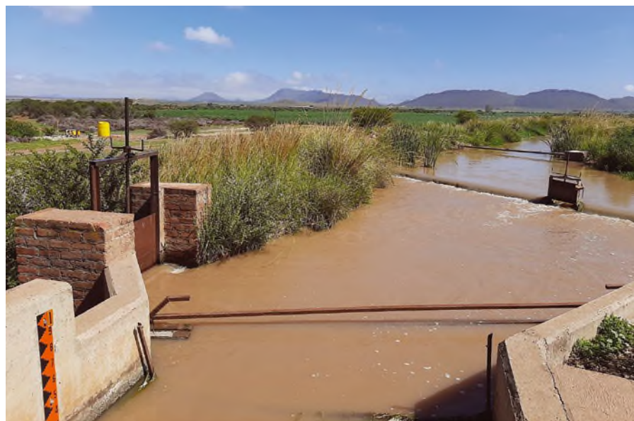
Canals and measuring devices in the Grassridge area within the Great Fish River scheme.
